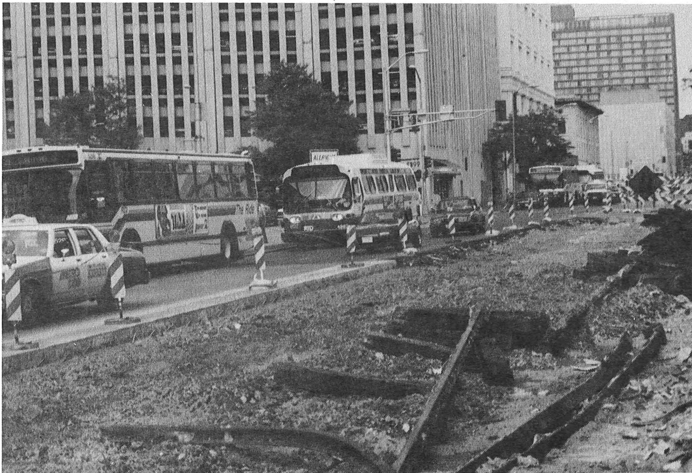
Modern RTD buses snake through the re-construction of the 15th Street roadbed between Stout Street and Champa Street in downtown Denver as old rails and ties from the streetcar era await their removal. Just out of the Central Loop, the old Route No. 64 streetcars turned north onto Stout Street in the background. (Joe Priselac Photograph)
